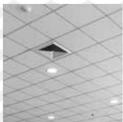
CEILING GRID FALSE CEILING
